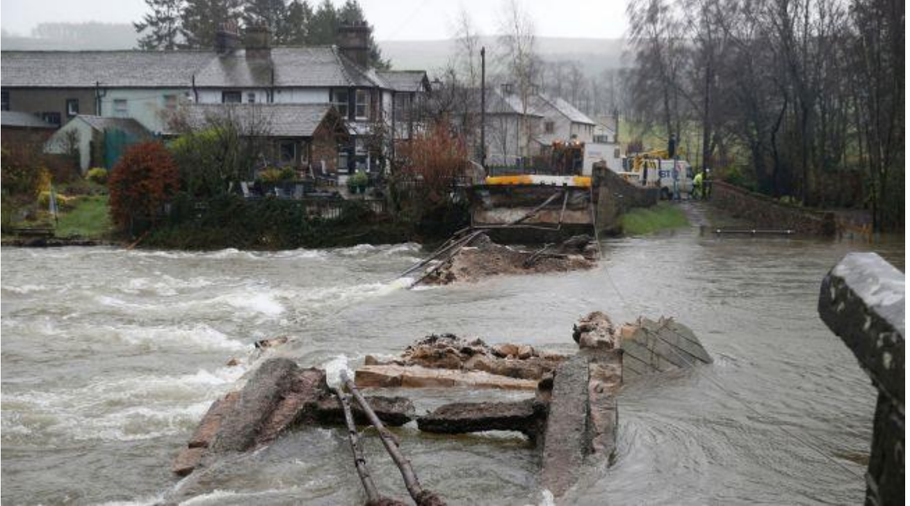
The clear up operation at Pooley Bridge after it was washed away by high water in December 2015.
